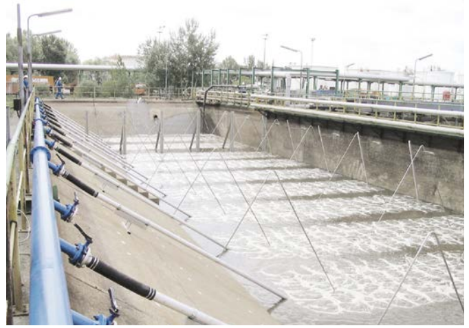
Sewage treatment plant Bayernoil-Raffinerie, Ingolstadt
