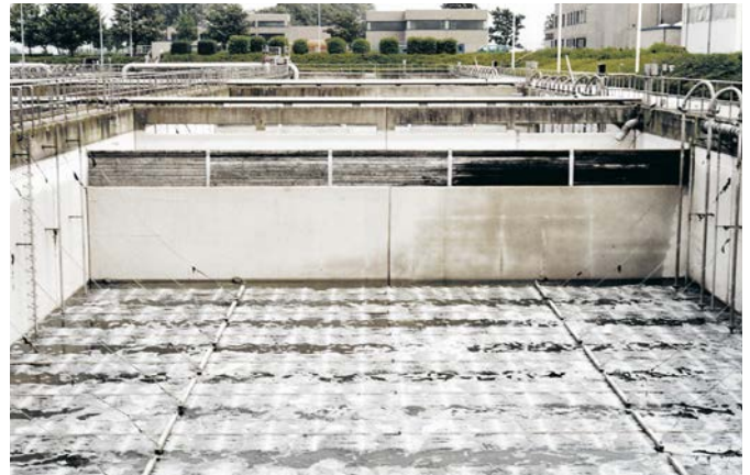
Sewage treatment plant Kleve, 180000 population equivalent
